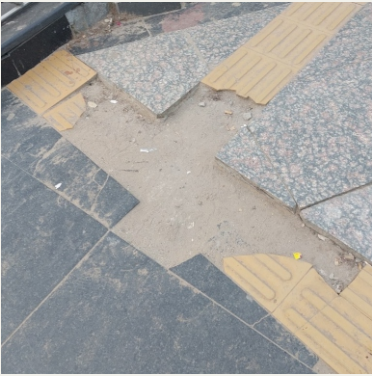
Prone to crack
